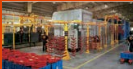
Robotically armed & conveyorized double booth powder coating plant with a capacity of 15 million sq inches / month
